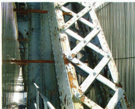
(top) Blasting and painting the bridge were well-contained, so traffic continued above and below the bridge.
